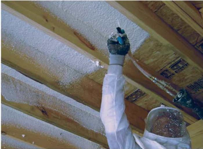
Spraying closed-cell foam into a garage ceiling cavity beneath a bonus room or bedroom.
